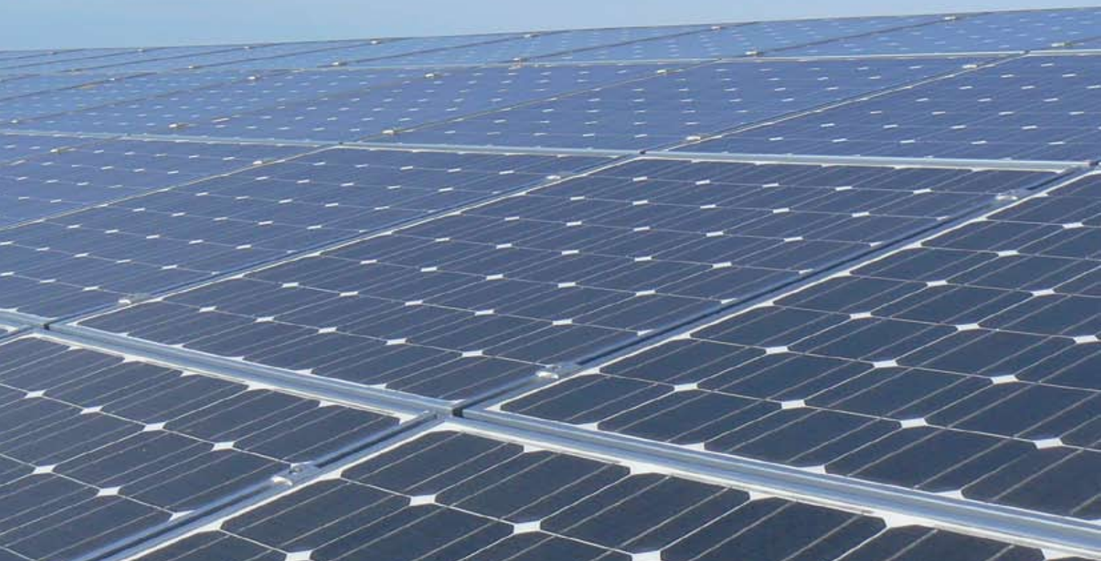
20kWp Solar PV on St Just Sports Centre
