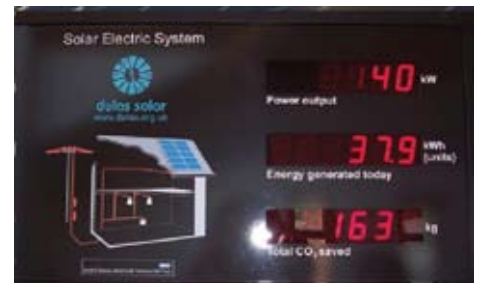
LED Display showing solar power being made and carbon being saved.
